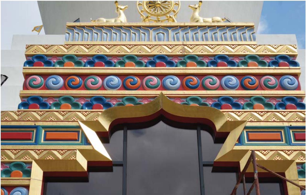
The splendor of the first completed gateway has been fully restored with a vibrant, colorful and ultradurable Kynar Aquatec®-based NeverFade® coating that will protect this architectural treasure for many years to come.
