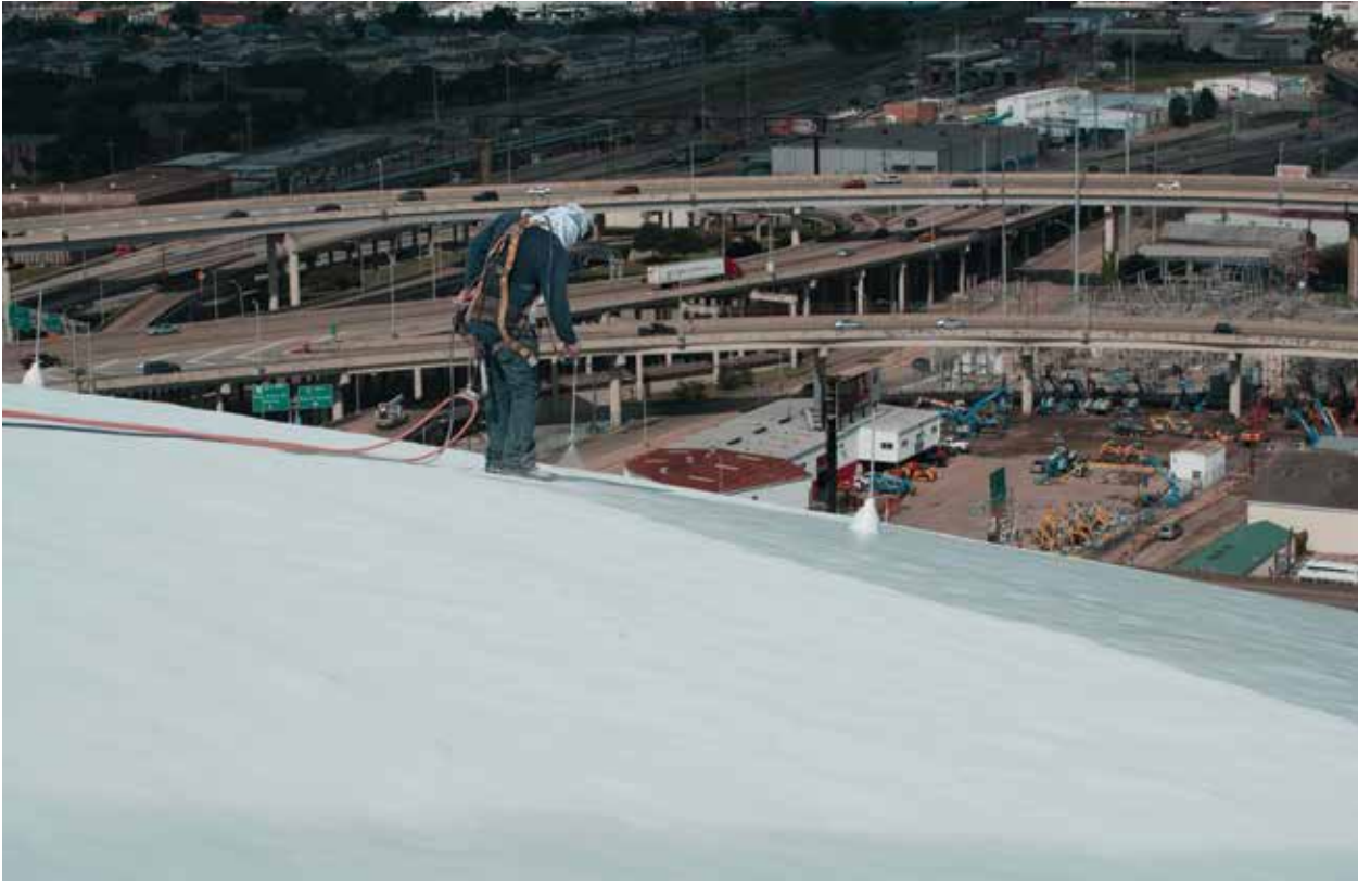
Workers sprayed on two Kymax® topcoats at a rate of 6 wet mils. This coating is designed to be weatherable and to have cool roof properties. Photo by Nationwide Photographers.
